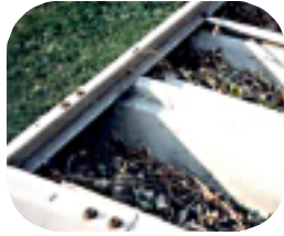
Out dated systems, such as this, allow debris to accumulate and are very difficult to clean.
